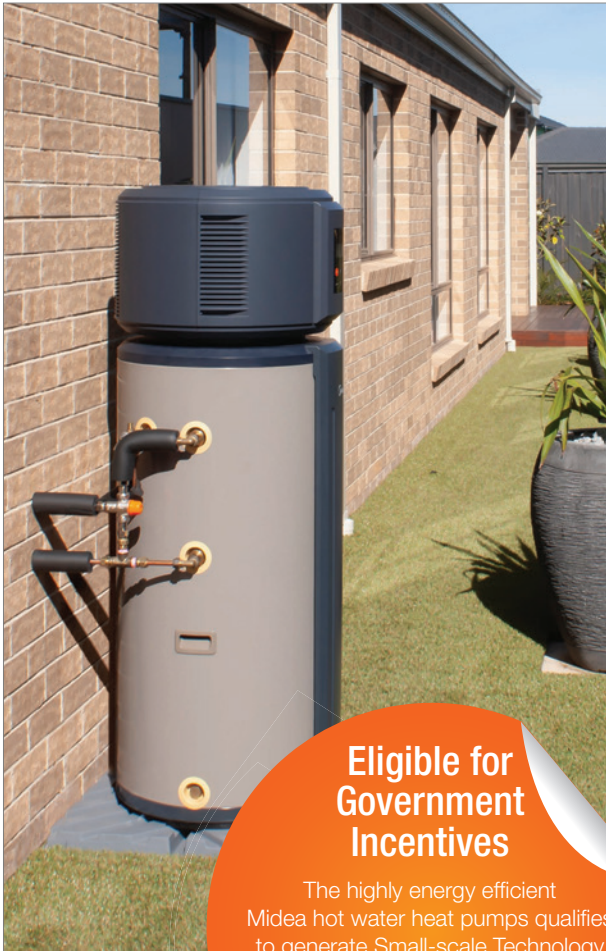
170L Installed Unit
